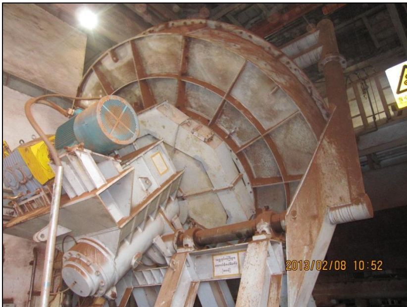
Flue dust prepare for recycling, Pelletizer
