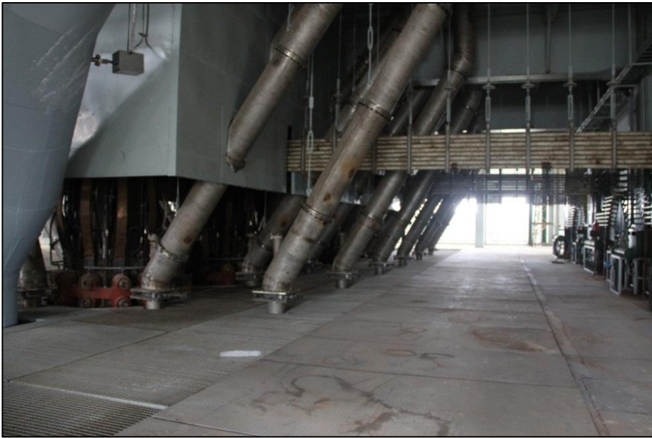
Electric Arc Furnace (2 nos.)
