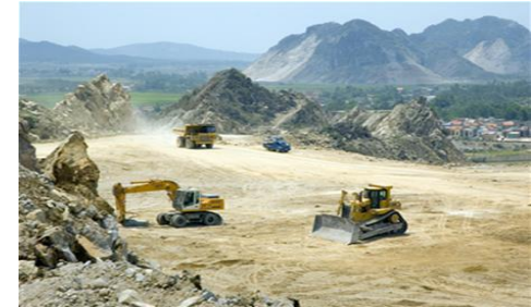
Blasting for leveling the top of the mountains in the limestone quarries
