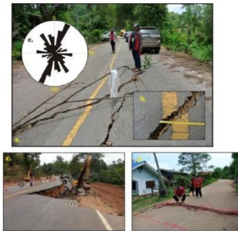
Fig.4 Ground crack was observed at Ban Mai Jad San, Dong Mada district, Mae Lao district, Chiang Rai province (a and b; see location 1 in Fig. 1). Highway and road were split by serious cracks on the highway 118 (Chiang Mai to Chiang Rai) at km 151–152(c; see location 2 in Fig. 1). Ground crack was also observed at Ban Huai San Yao, Dong Mada district, Mae Lao district, Chiang Rai province (d; see location 3 in Fig. 1). Principle orientation of ground cracks shown as a rose diagram (e, inset in a)
