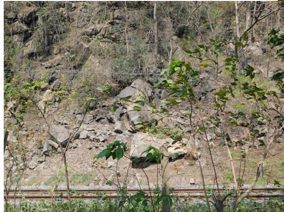
Rock fall next to railway in Muak-Lek District, Saraburi (0728572E 1620547N)
