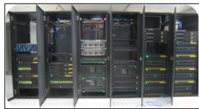
Computer cluster in data processing center
