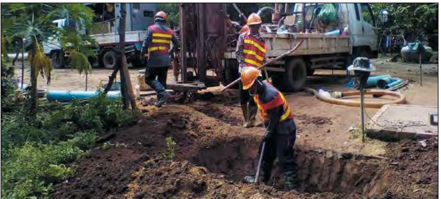
Drilling and Monitoring Site at Preak Thouch, Preak Tlorb , Lerk Dark Kandal Province, Cambodia.
